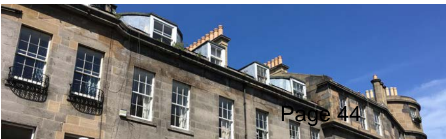
pic.3d: array of historic zinc-clad dormer windows, various forms, to the front elevation double hipped roof 4,6,8, Barony St.
