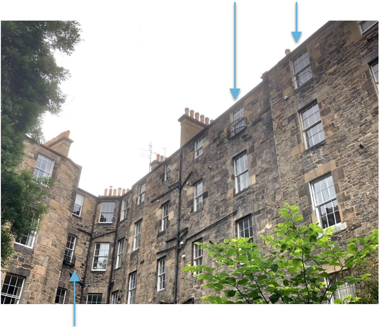
“juliette” balcony to rear elevation of flat 2f2, 2 Barony Street, directly below flat 3f3.
